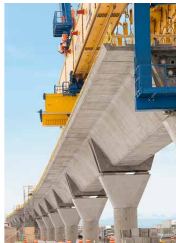
More than a third of the metro runs as an elevated railway on pillars. Concrete elements are joined together with the assistance of Sika's high-performance structural adhesives.
