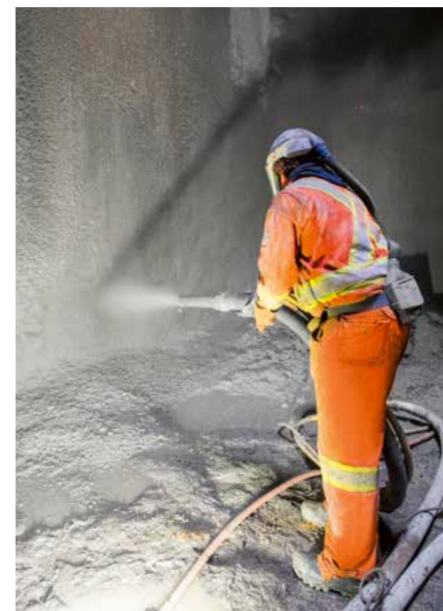
In the center of Montreal, the new light rail network is mainly built underground. Directly following excavation, the tunnel walls are secured with Sika's shotcrete.
