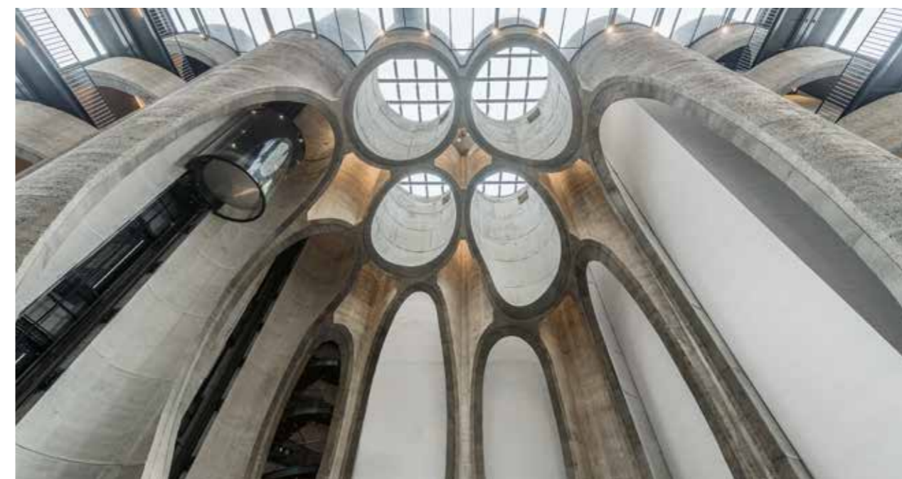
The grain silos of the Zeitz Museum have been made a dazzling feature by the architect Thomas Heatherwick. Sika provided the state-of-the-art solutions to restore the concrete and preserve the building structure.
