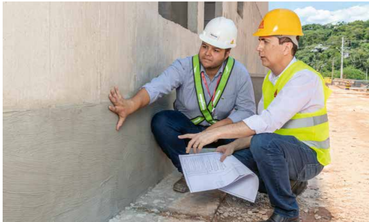
In addition to a high-quality product portfolio, Sika's strengths also include advising the client on the building site. Together with Direcional Engenharia, the best solutions for the specific project requirements were defined and implemented.
