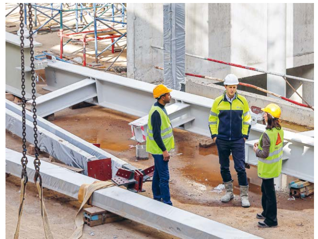
The striking skyscraper has to meet stringent requirements. Sika is involved in the project with various products and know-how.
