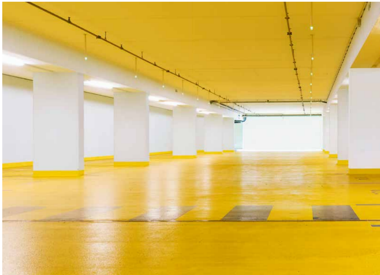
The parking garage at Linz Main Station in Austria was refurbished in record time.
