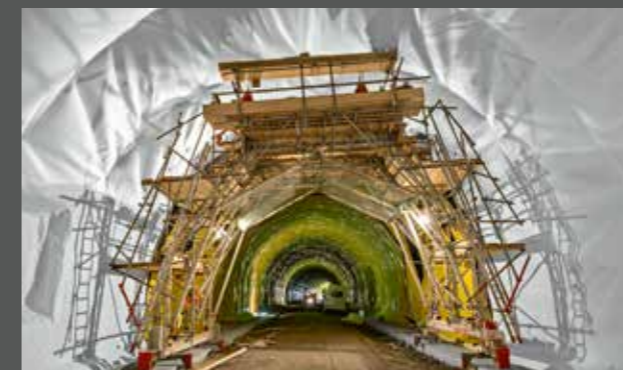
120,000m 2 of Sikaplan® waterproofing membrane is being used in the construction of the Brenner Base Tunnel. On completion, the 55 km long tunnel between Austria and Italy will be one of the longest underground railway connections in the world.
