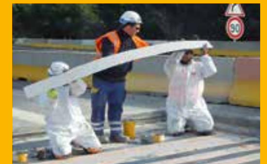
The reinforcement work had to take place with the highway open to traffic. Sika provided training for applicators and supported the project with technical advice.
