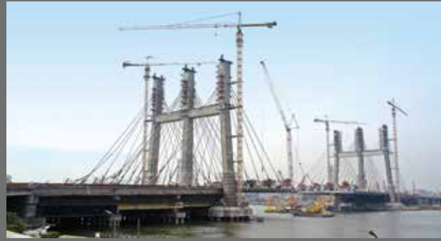
In the construction of the Rod-Al-Farag bridge in Cairo, Sikagard®-550 W Elastic system is being used to protect 600,000 m 2 of concrete from carbonation as well as Sikacrete®-114 free flowing micro-concrete grouting. Upon completion the bridge will be comprised of six lanes in each direction as well as two lanes for buses and a metro line.
