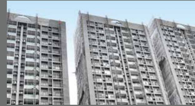
Sika is supporting the facade refurbishment of 19 blocks of high-rise buildings in Hong Kong by providing sealing, bonding, and waterproofing systems. In many large cities there is a great need for repair and maintenance of buildings and infrastructures. Renovation of building envelopes improves energy efficiency, durability, and safety.
