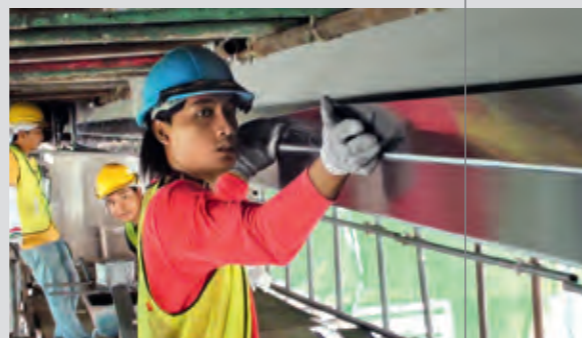
The first Penang Bridge was strengthened and overhauled without closure to traffic using Sika Refurbishment solutions.
