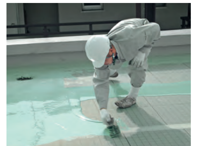
Global quality, local application: Sika transfers skills and know-how directly on the spot.
